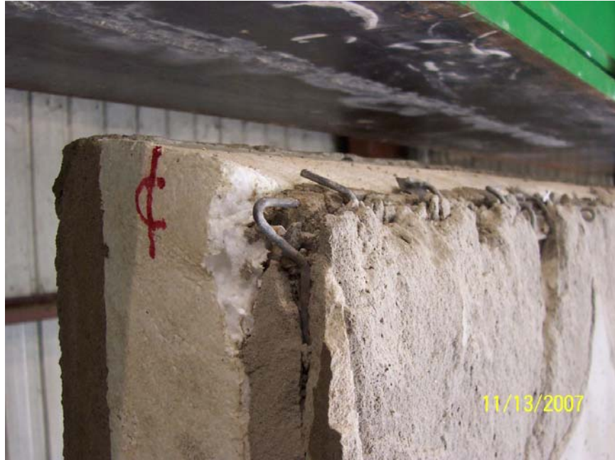
Figure 10A: 4X14A1 Failure mode at top of wall
