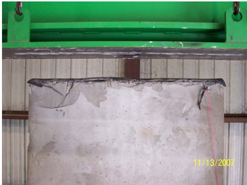
Figure 11A: Rear view of failure mode
