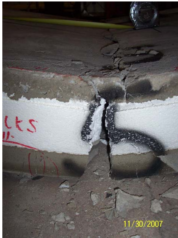
Figure 8A: Failure mode (close-up)
