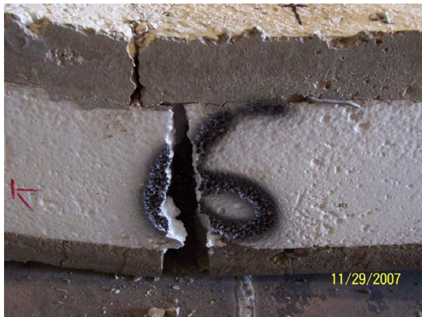
Figure 8A: Failure mode (close-up)
