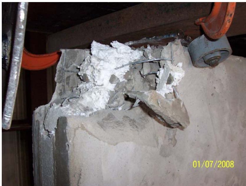
Figure 6A: Failure mode (close-up)
