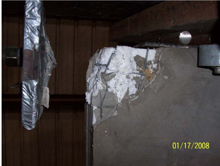
Figure 9A: 8X14S3 Failure mode
