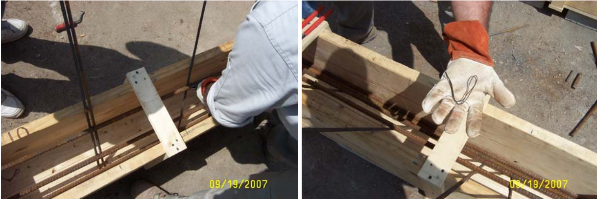
Figures 4 and 5: Installation of #5 rebar into wooden footer mold using 1/8" rebar tie wire
