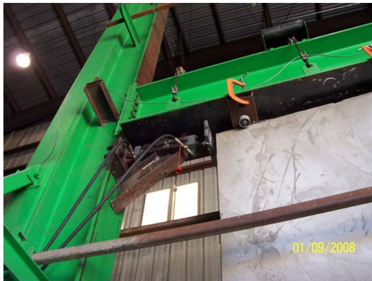
Figure 23: Hydraulic cylinder connection to racking frame
