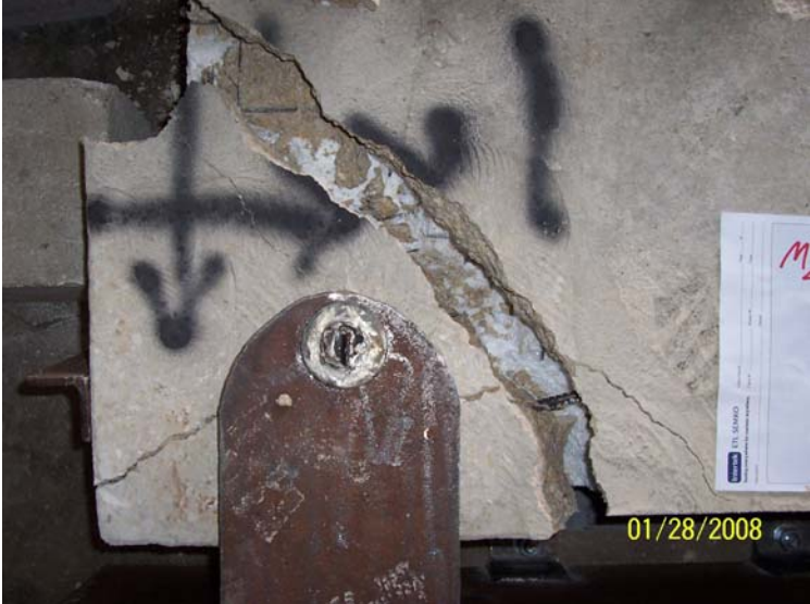
Figure 5A: Failure mode at hinge
